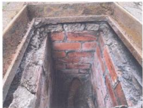
P8 Manhole Showing mortar seating destroyed
