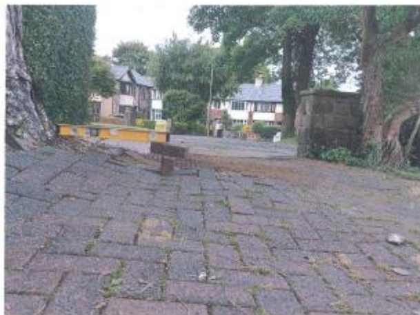
Crossfall on drive caused by tree root Growth at foot of Pine tree
